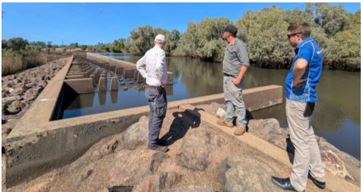
High-performance fish ladder at Glenore Weir
